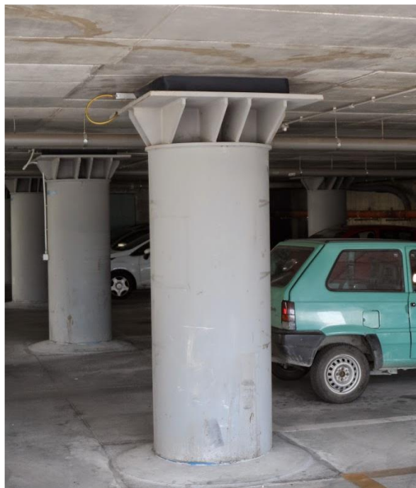
Figure 6. Base-isolation of a residential building in L'Aquila, Italy (courtesy of D. Pohoryles)
