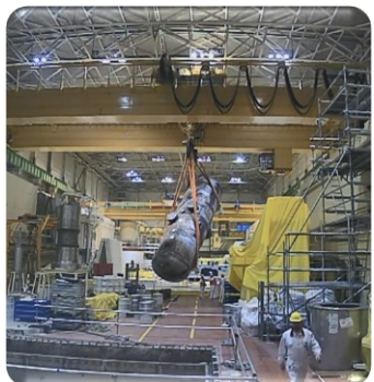
The existing crane in the reactor hall was modified for also for the transport needs of SGs
