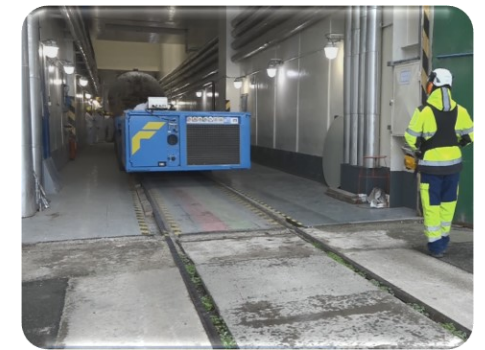
Individual SGs were transported from SG boxes to the siding corridor of the reactor building (loaded onto a special truck )
