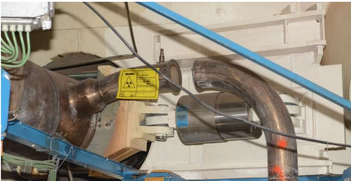
Figure 10: Modification of the blind pipe of the low-pressure emergency filling of the primary circuit.
