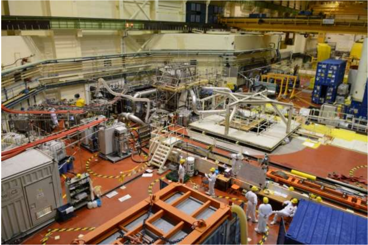
Figure 7: DFD line at Unit 2 V1 NPP.
