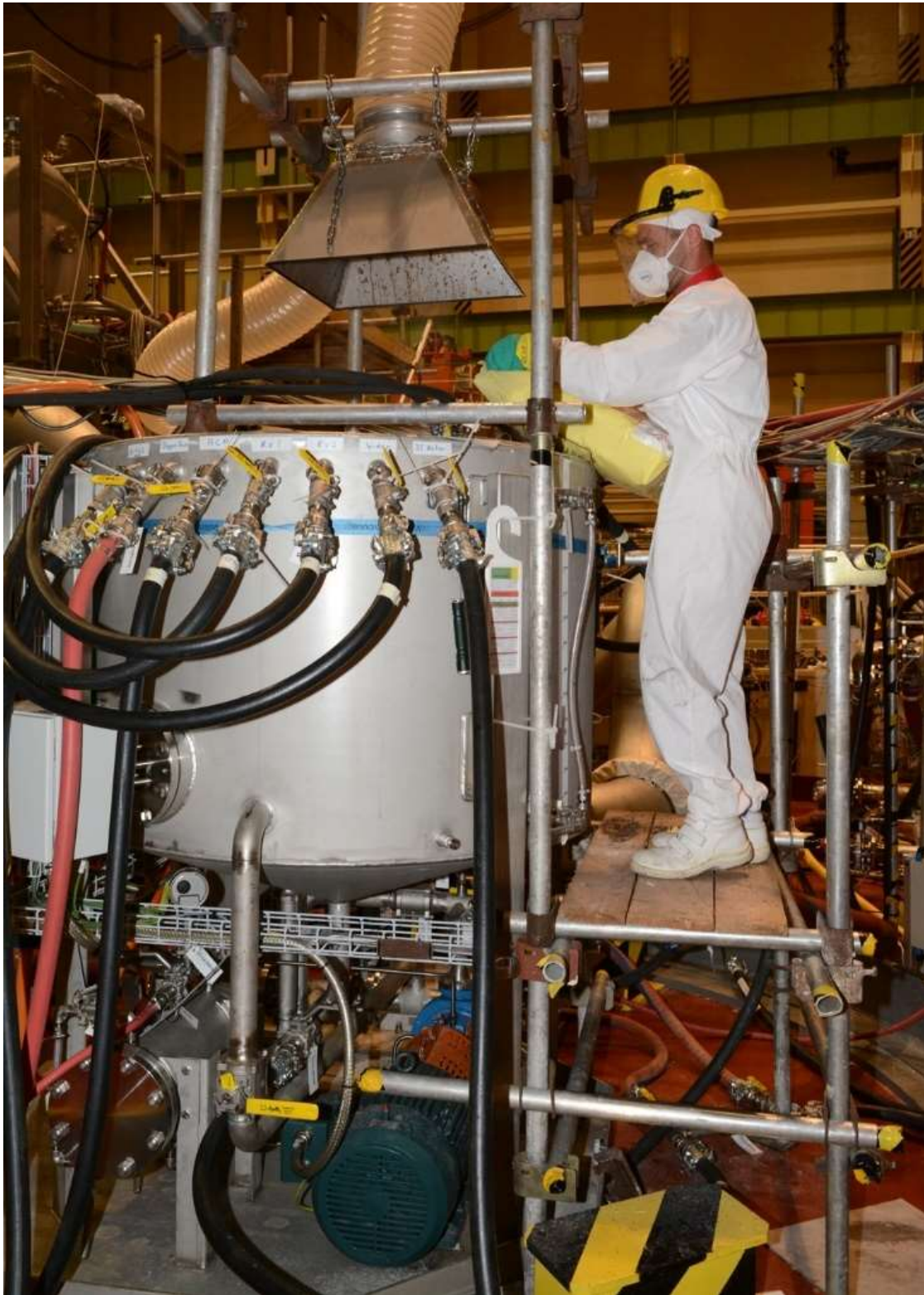
Figure 6: Chemical dosing into the Venting/Mixing Tank.
