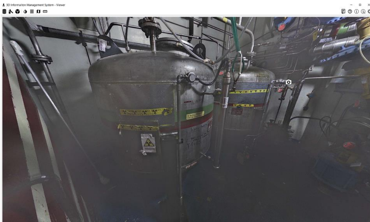
Figure 20: View of tanks in bunker 1106 in 3DIMS
