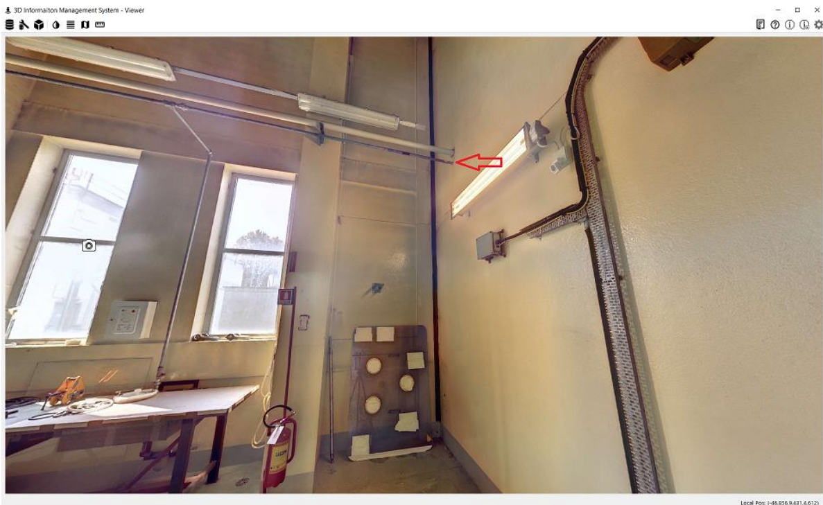
Figure 28: Continuation of the same pipe in room 4413 of ADECO, here the system is identifiable by colour coding the penetration is again marked with a red arrow
