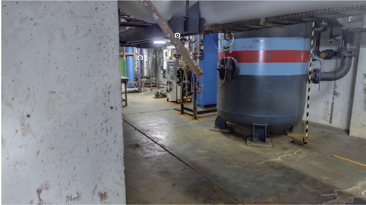
Figure 8: 3DIMS view after double-clicking and jumping to the new scanning position “20180227_Ed83_-6.0m_Loc4218_Scan6” in room 4218 of ADECO (building 83) (source 3DIMS software)
