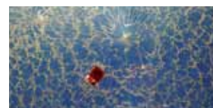
Crack in laminated glass.
