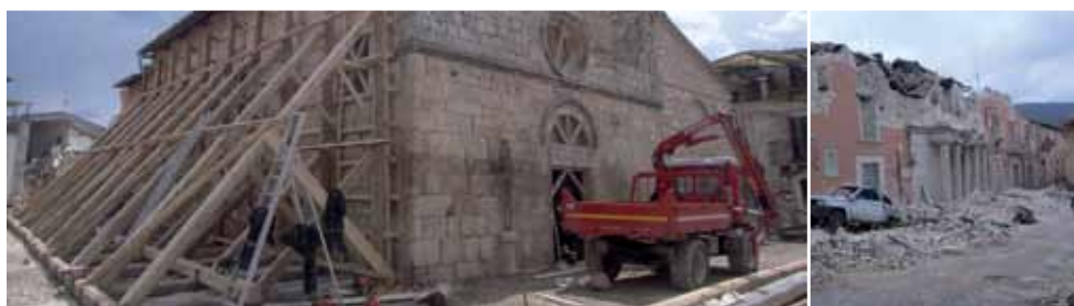
Left: Propping up the San Paolo Apostolo Church in Onna; right: Damage to the Prefecture building in L'Aquila.
