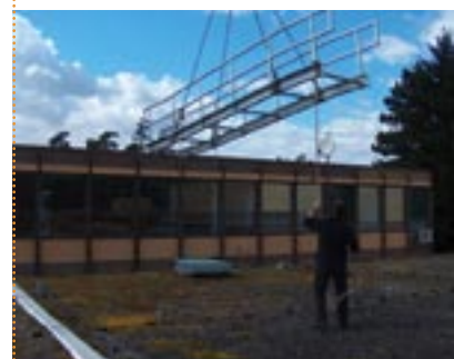
Fire protection at JRC-ITU: Installation of a new emergency evacuation bridge for the administration building
