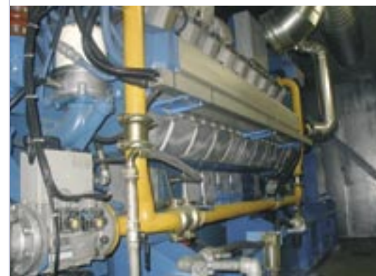
Ispra cogeneration plant.
