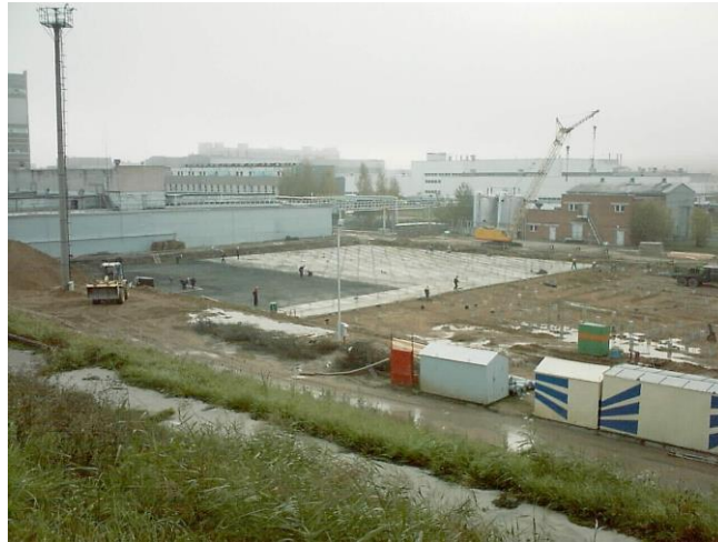
Figure 5-1. The construction works were performed by local contractors' organizations under separate contracts with INPP in less than 1 year.
