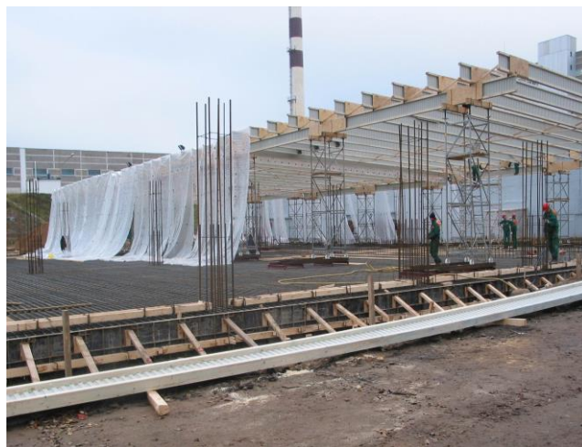
Figure 5-2. 1250 vibropiles were driven under the foundation slab. The foundation slab was concreted continuously for 10 days during the cold season.
